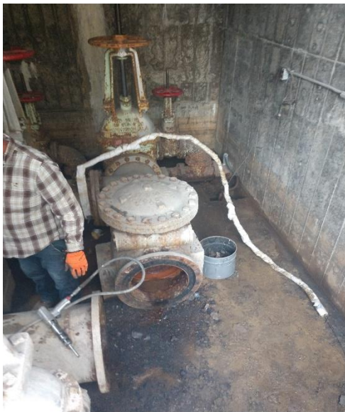
Dirt Dawg Excavating is changing the valves inside the valve house at the City's underground reservoir.
