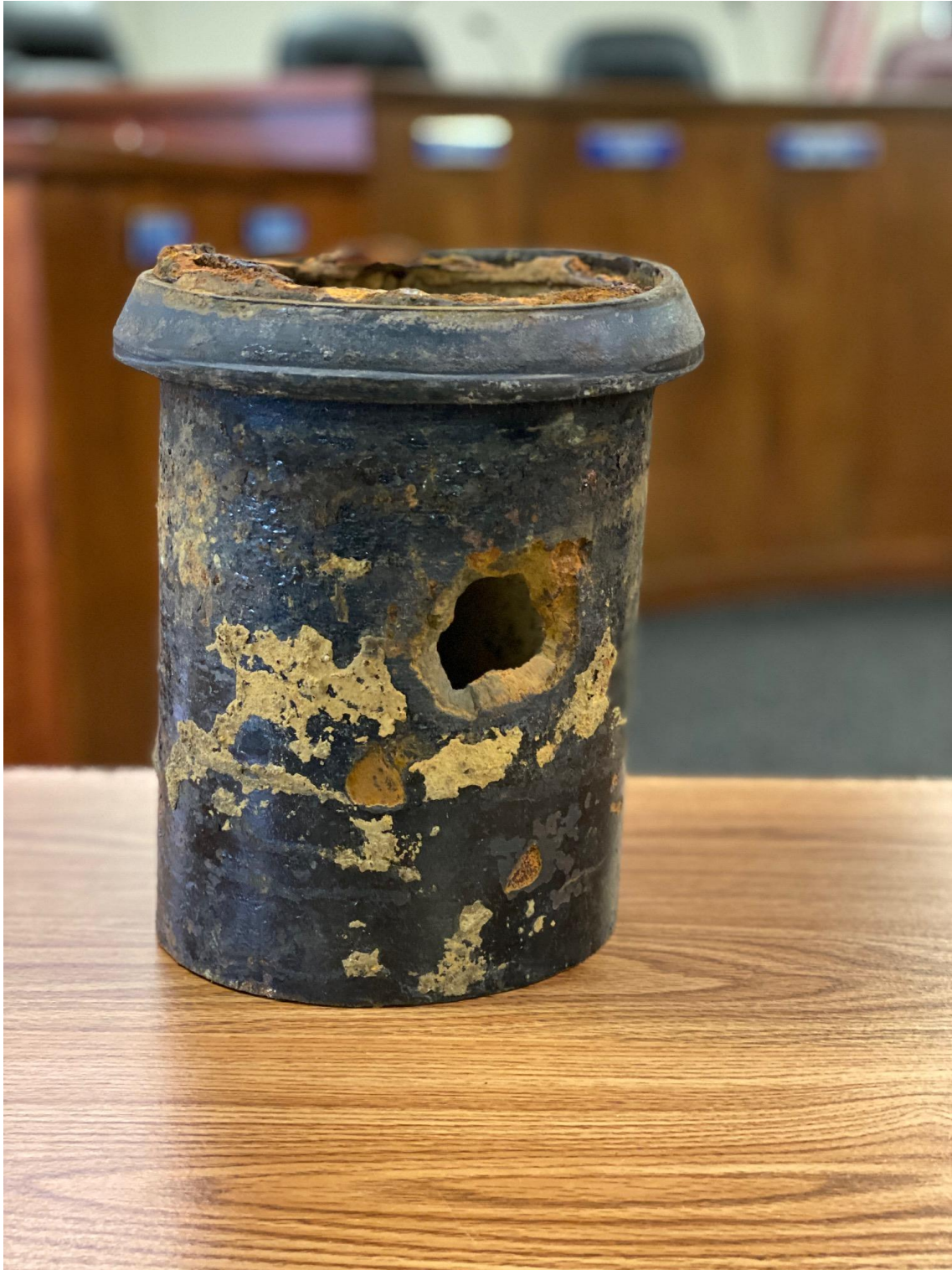
A section of one of the water lines was pulled and replaced at the north end of Mount Vernon. The original pipe was installed in 1962 and has given way to corrosion. Mount Vernon crews continue to repair or replace the water lines as they update fire hydrants and watch valves.
